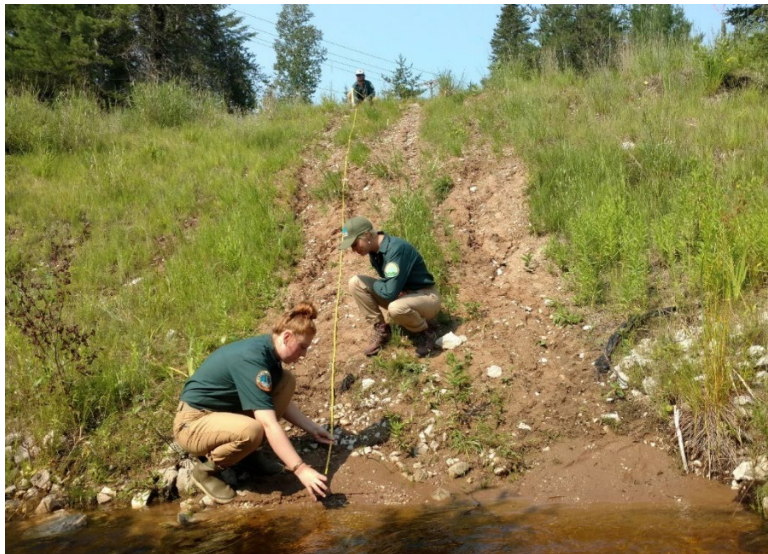
Photo: GLCC field technicians assessing erosion at an unregulated stream ford
