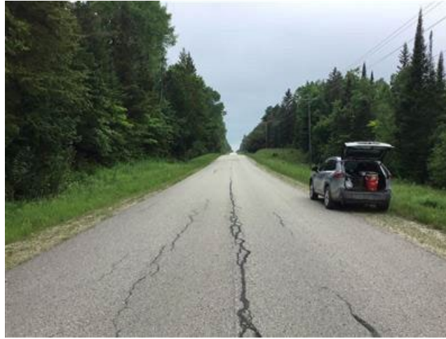
Right approach to crossing
