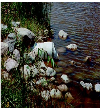
Typical Outlet Pipe
